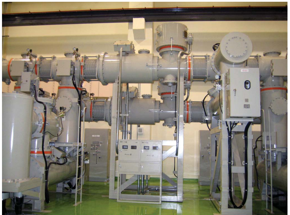
三相共管 161KV GIS (3phase common enclosure)
