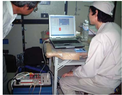
電驛測試保養 Relay test and Maintenance
