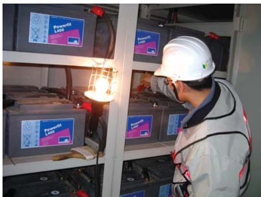
UPS電池保養 Maintenance
