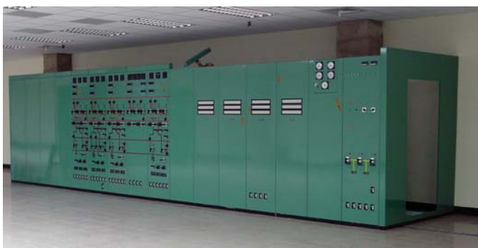
遙控及保護電驛盤 Remote Control and Protective Relay Panel
