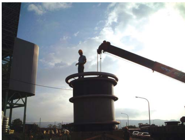
161KV GIS 遞昇加壓 161KV step up withstand voltage test
