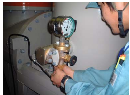
氣體壓力表測試保養 SF6 GAS Density Switch test
