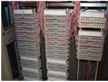
通信線線架 Communication Terminal Rack
