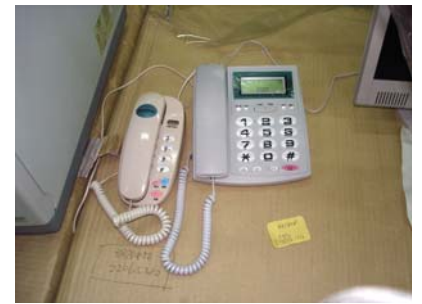
主變電所防情、調度電話 Security and Operation Command Phone
